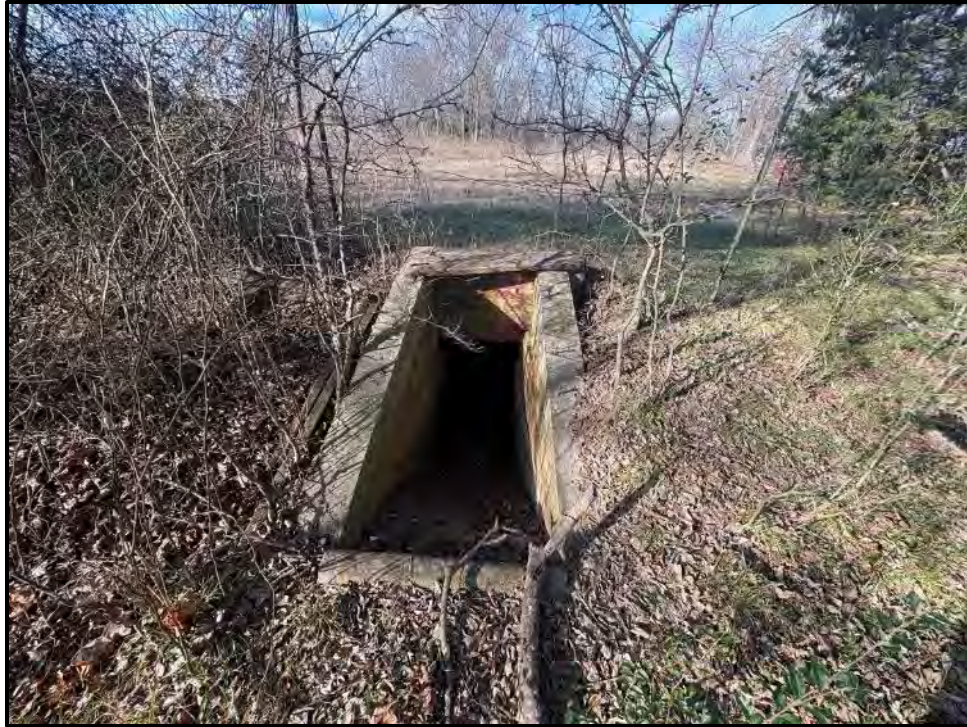
Photo 5. Brick basement entrance near the dilapidated residence in Photo 6.
